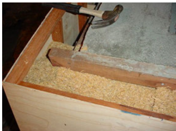
Figure 1. The external wall cavity of the simulated building filled with dried rice husk.
