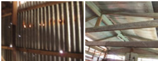
Fig. 11. (a) Leaking galvanized iron roof (b) Distressed wooden beams
