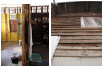
Fig. 12. (a) Decaying wood column (b) Distressed wooden wall
