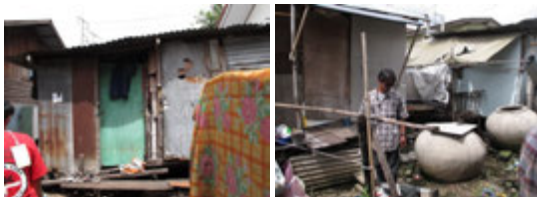
Fig. 13. (a) Distressed galvanized iron wall (b) Deteriorated environment
